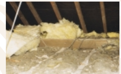
This image shows the additional layer of mineral fibre missing over a substantial portion of the attic.
