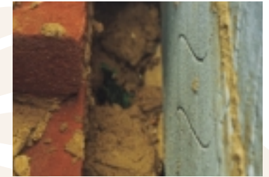
This image shows the accumulation of mortar on the top surface of mineral fibre full fill batts amongst other elements of poor workmanship.
